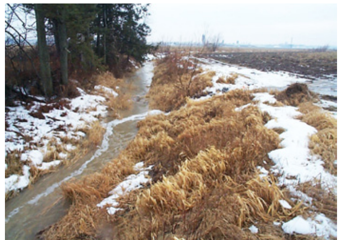
Photo 5 : Turbulence at outlet apron of rock chute spillway Source : Ghislain Poisson (MAPAQ)
